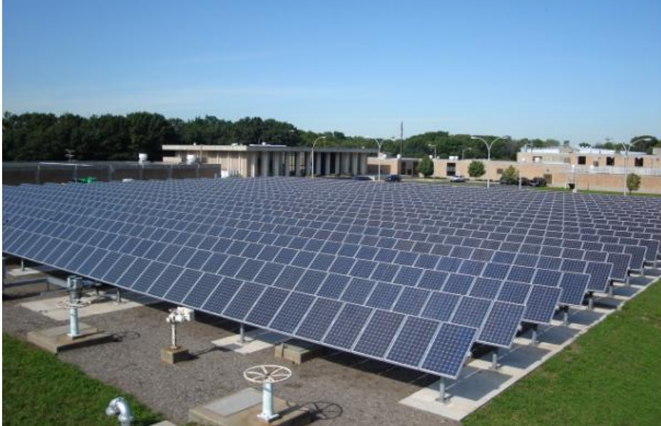
Solar Panels at Our Largest Treatment Plant
