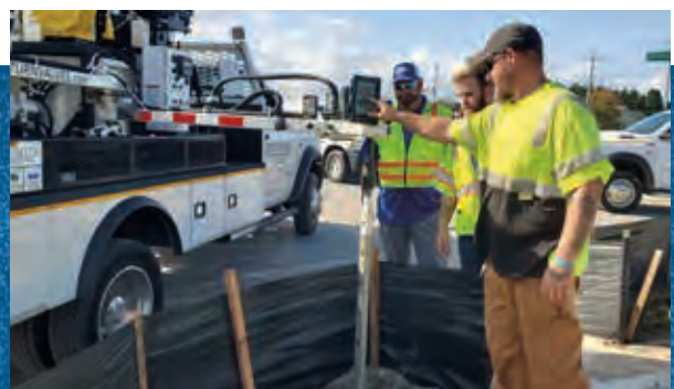
The team at Tidewater Utilities, Inc. works to interconnect water systems which helps maximize system efficiencies.
