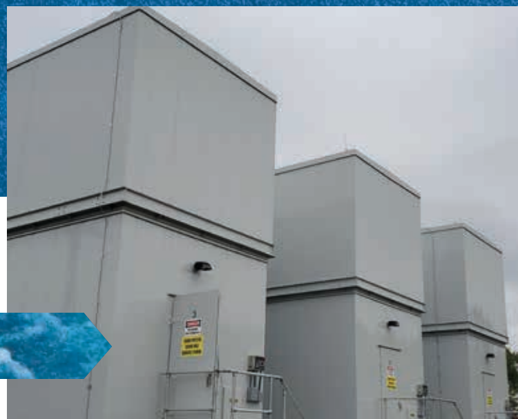
New generators help maintain consistent operations during power outages.
