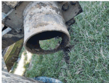
Aging Influent Piping
